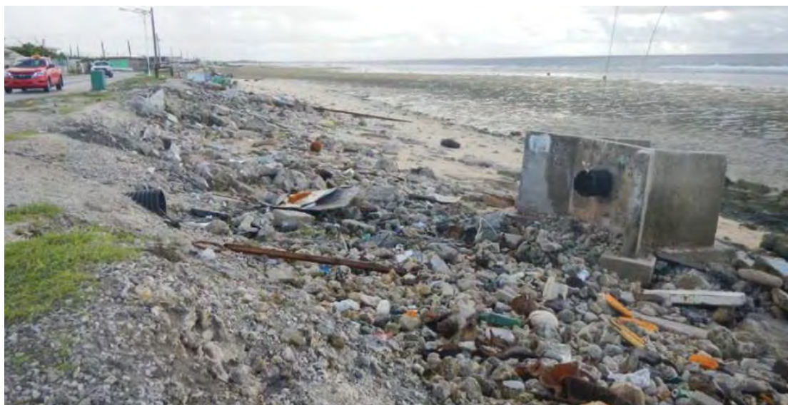
Figure 2-7: Erosion and failure of the storm water outlet 15
