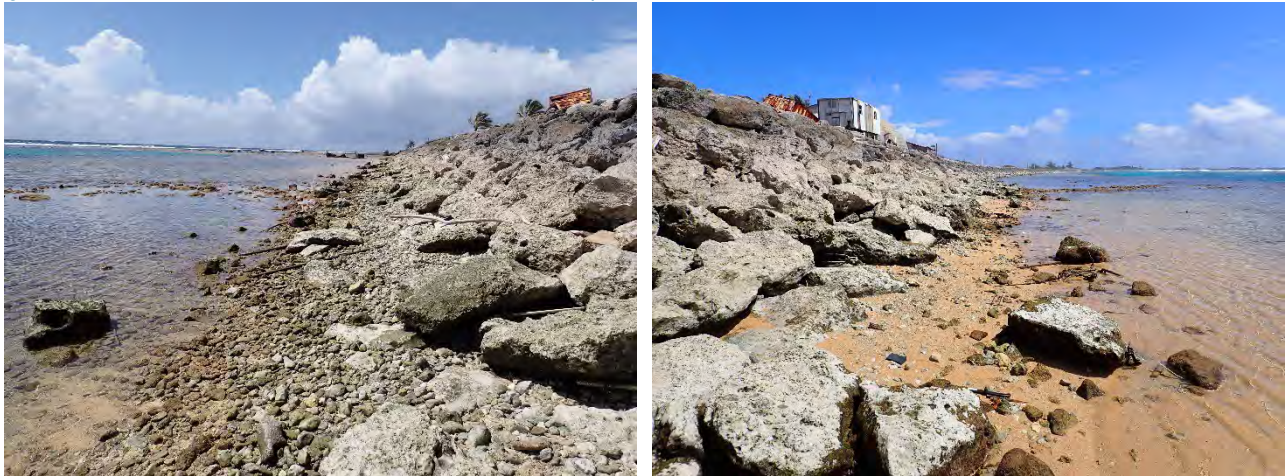
Figure 4-1 WCR Condition – Shows toe failure and displacement
